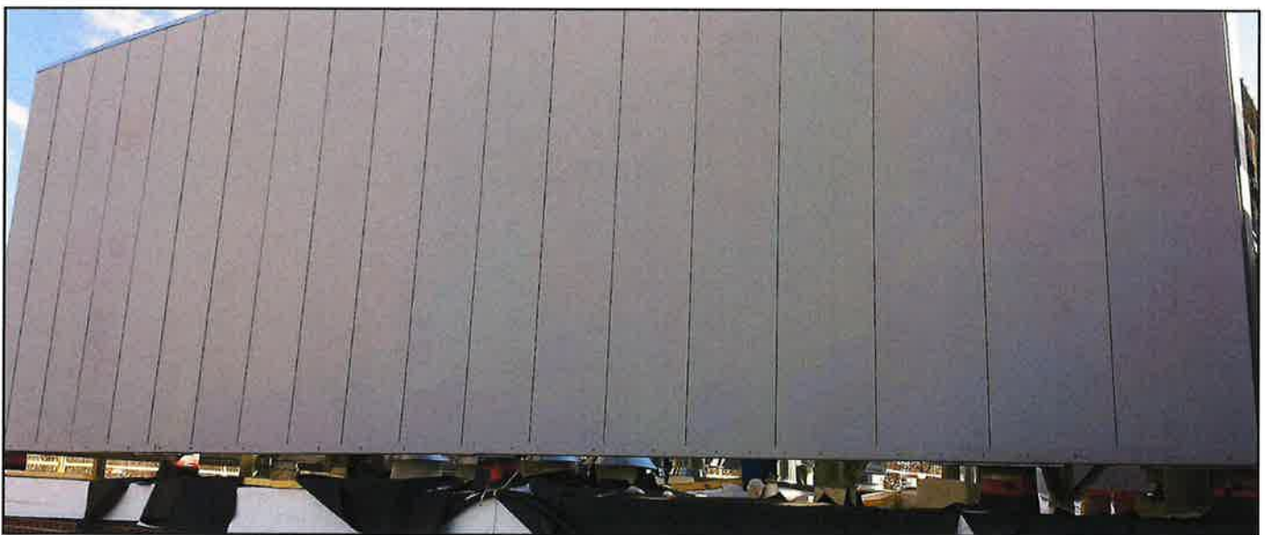
NOISEBLOCK™ rooftop barrier wall surface mounted to structural support steel
